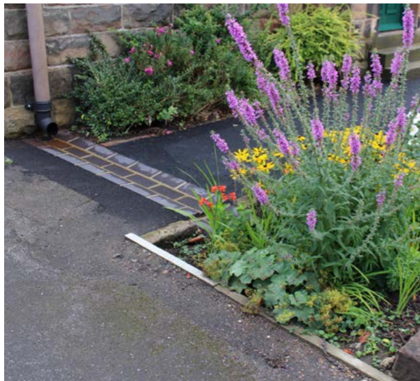
Image above: A retrofit downpipe shoe and brick channel into a rain garden.
