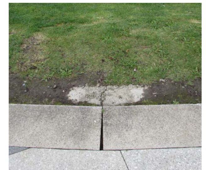
Image below: Example of topsoil washout. The haunching is set near the top of kerb allowing for minimal topsoil to be placed, therefore prone to erosion over time. Credit KCC
