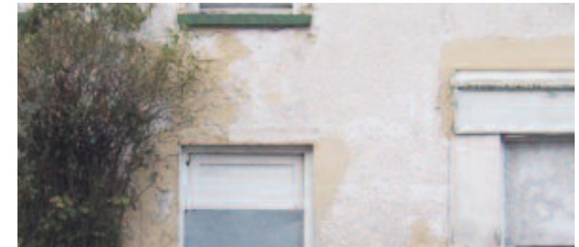
Example of a building in need of repair
